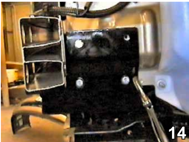
14. Insert the nutplate into the opening on the bottom of the frame (see photo 13) to align with the upper drilled hole on the driver's side, tighten the lock washer and hex nut.
